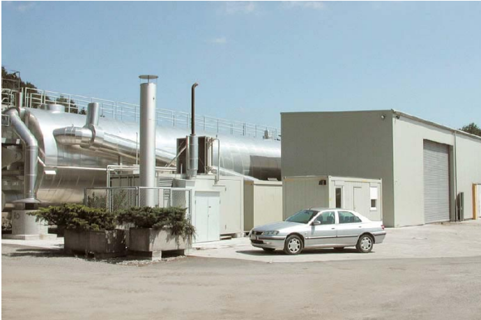
Biogas Plant in Switzerland
