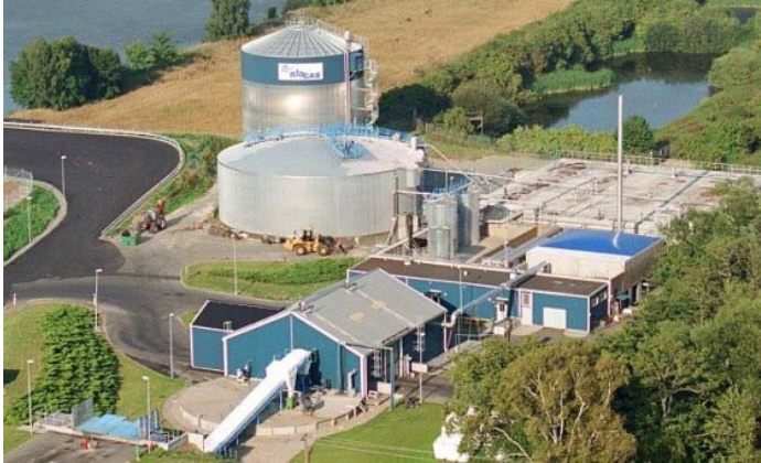
Biogas Plant, Kristianstad Municipality, Sweden
