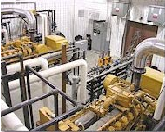
Cogeneration at the Lethbridge sewage plant
